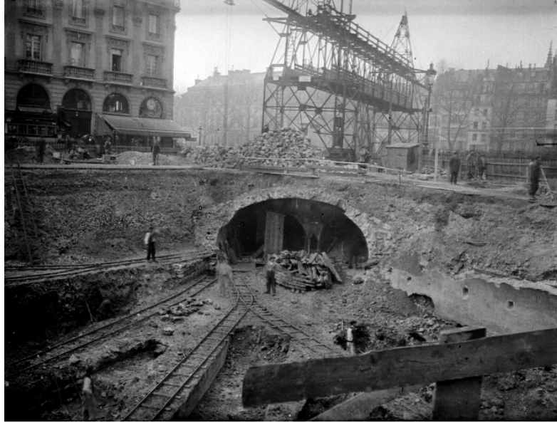
(fig. 4) Paris Métro Under Construction 1902-1910. The tracks were dug at street level in the open air and covered over later. Web. http://en.wikipedia.org/wiki/File:Paris_Metro_construction_03300288-3.jpg . Dec 30, 2009
